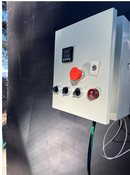
Figure 33: Control System Attached to Powder Coating Oven
