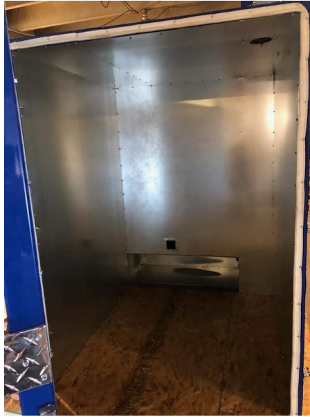
Figure 15: Exhaust System for EPTEX
